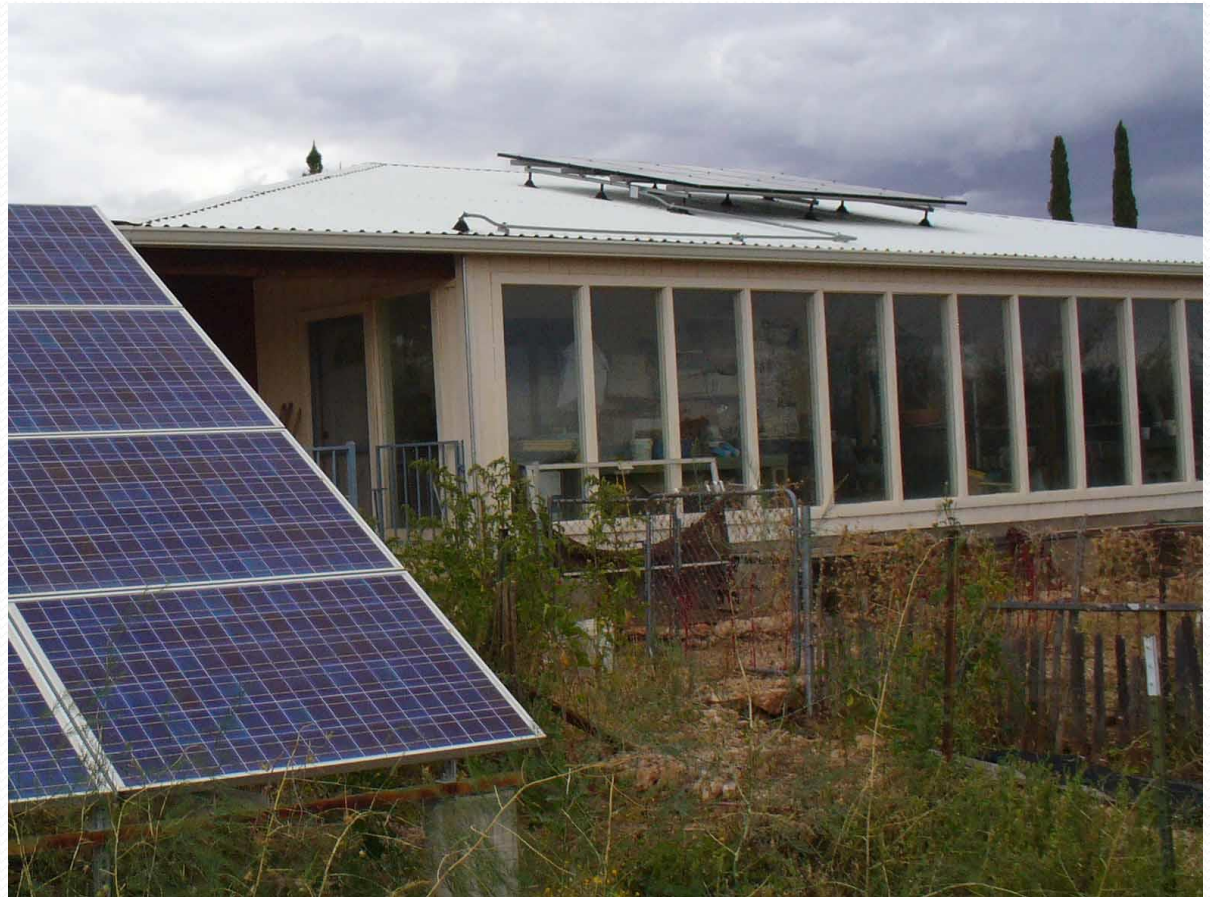
3.5 KW Solar Arrays
